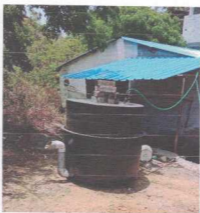
Figure 4.1: Bio gas plant
