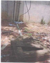
Figure 6.2: Rain water collection system
