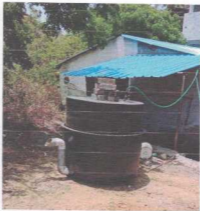
Figure 4.1: Bio gas plant
