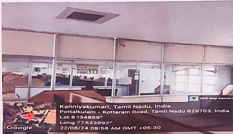
CCTV CAMERA AT COMPUTER LAB
